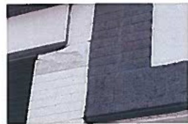
A large percentage of the brick surfaces in the HCD have been painted. Avoid painting masonry or using abrasive cleaning techniques.
